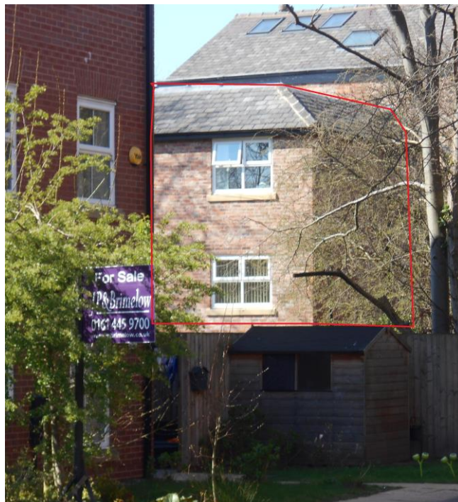
Unauthorised rear extension as viewed from Besford Close
